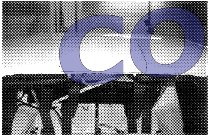
PHOTO No.117 FLAPS FOR VENTILATION
